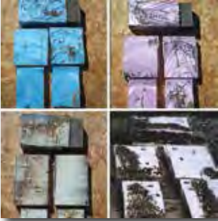
Termite-Damaged Untreated Foams
